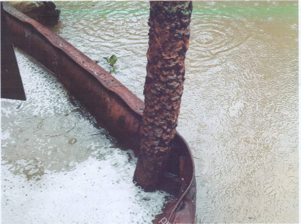
Picture showing Corroded flow line on exposure with boom deployed.
